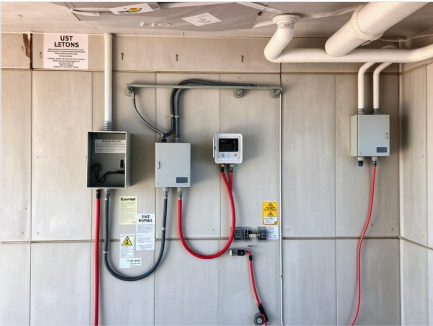
Item 03 — grounding bonded at junction boxes Aug 11, 2026 02:33 PM MDT · 40.3916, -111.8508
